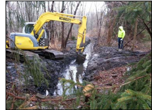
Division of Mosquito Control staff use equipment to remove sediment from a ditch. This increases flow and reduces flooding.
